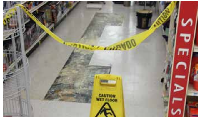
... and causes downtime and high repair costs
