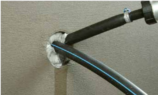
KÖSTER KB-Flex 200 is installed into the void using the KÖSTER Special Caulking Gun.
